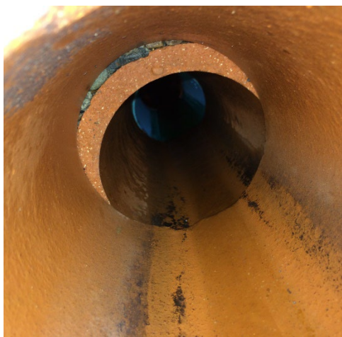
Offset Joint Detected via TV Inspection
