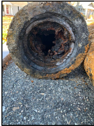
Old Unlined Cast Iron Water Main Pipe
