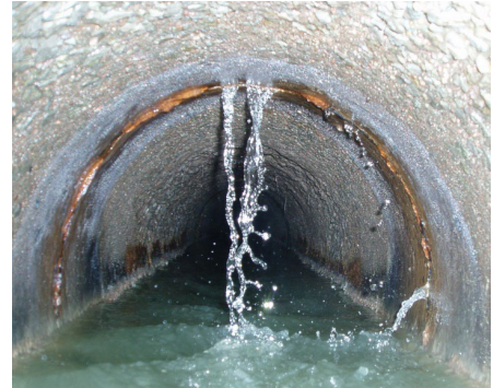
Infiltration into a Sanitary Sewer
