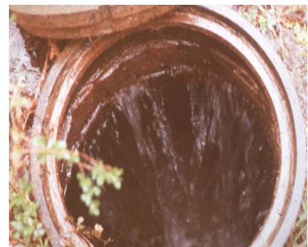
Inflow into a Manhole during Flooding
